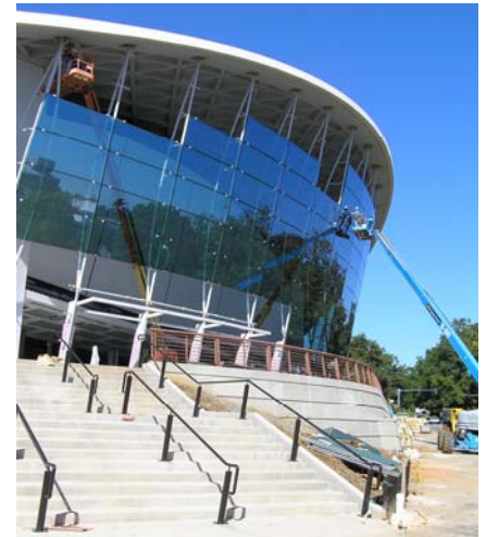
Contractors are installing nearly 350 glass panes, each weighing about 1,200 pounds, for a total of 210 tons of glass in the new renovation.
