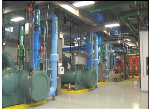
UGA's new District Energy Plant No. 1 serves as a model for energy and water conservation.
